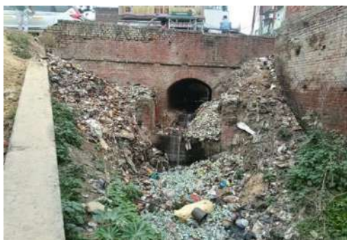
Image 4-4: Solid waste accumulated at Banka drain
