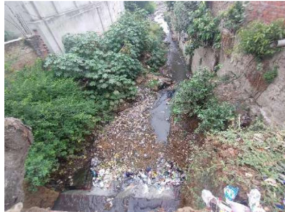
Image 6-8: Solid waste blocking flow at Roshan Ganj drain I&D
