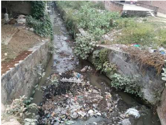
Image 6-7: Solid waste blocking flow at Yunus Khel drain
