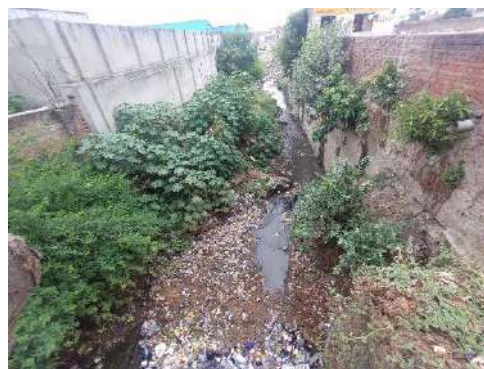
Image 4-5: Solid waste accumulated at Roshan Ganj drain into the Khannaut river
