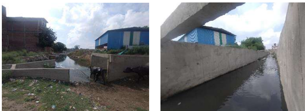
Image 6-1: Sewage outflow along with minor drain after intercepting the Lodhipur drain
